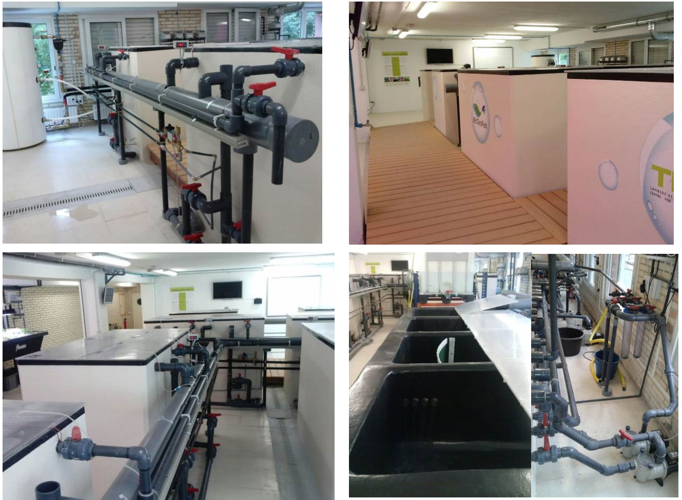
Figure 1. Culture Tanks (H1-H4) and the four compartment cleaning system (R1-R4).
